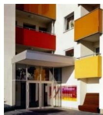
Figure (9) Renovating the building's elevations and covering them with a thermal insulation system with light beige and red paint
